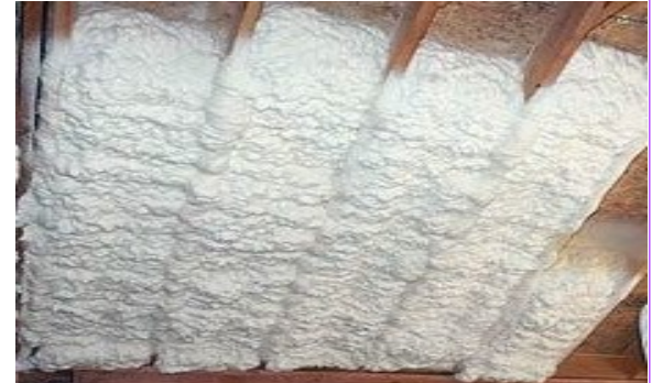
Spray foam is applied directly to the underside of the roof making a "Hot Roof" – No ventilation is installed
