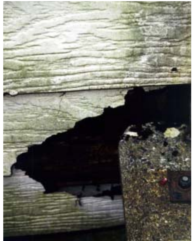
Another common problem is a lack of flashing and/or details that allow water to enter the siding
